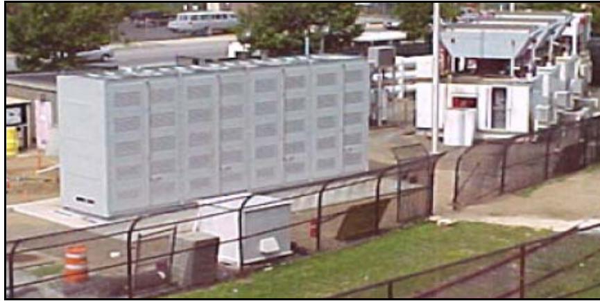
Figure 4-10 NYPA 1.2-MW/7.2-MWh Sodium-Sulfur Battery Facility
